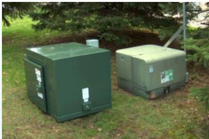
Community Energy Storage – 80 CES units servicing appx 350 participants (reduced to lab testing of 4 units)
